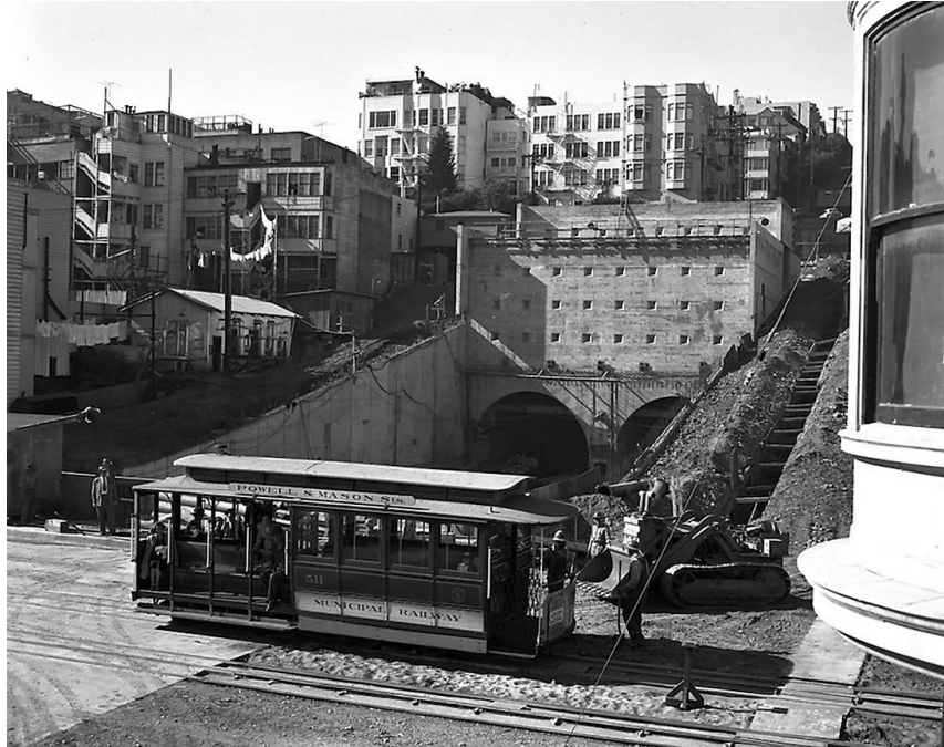
Construction of the Broadway Tunnel at Powell Street, November 5, 1951. (SFMTA Photographic Archive, as cited in Cordova and Lammers, 2018)
