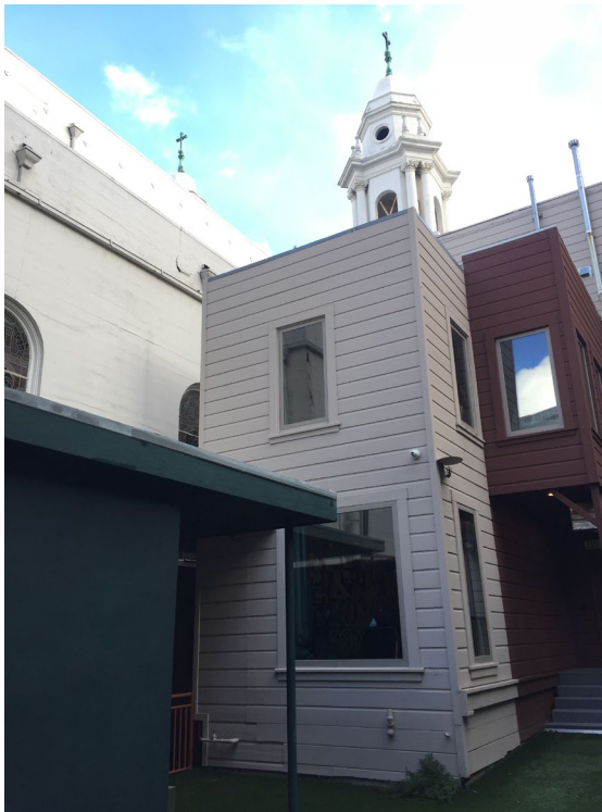
A portion of the adjacent property (908 Broadway) encroaching into the rear side yard of the subject property, view southeast.
