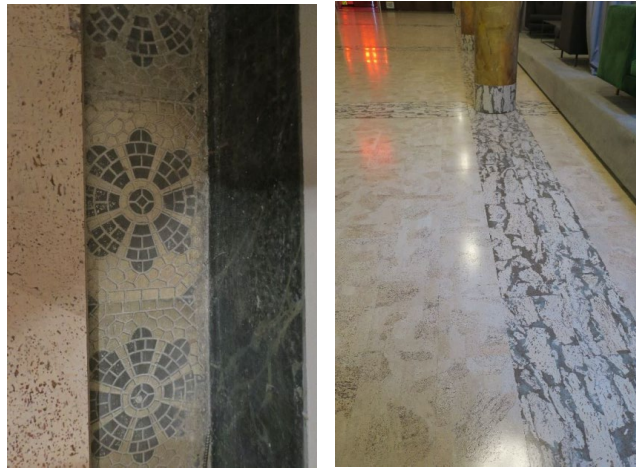
Tile flooring beneath cork flooring (left). Faux-marble cork flooring covering original tile and wood parquet flooring (right). (Page & Turnbull)
